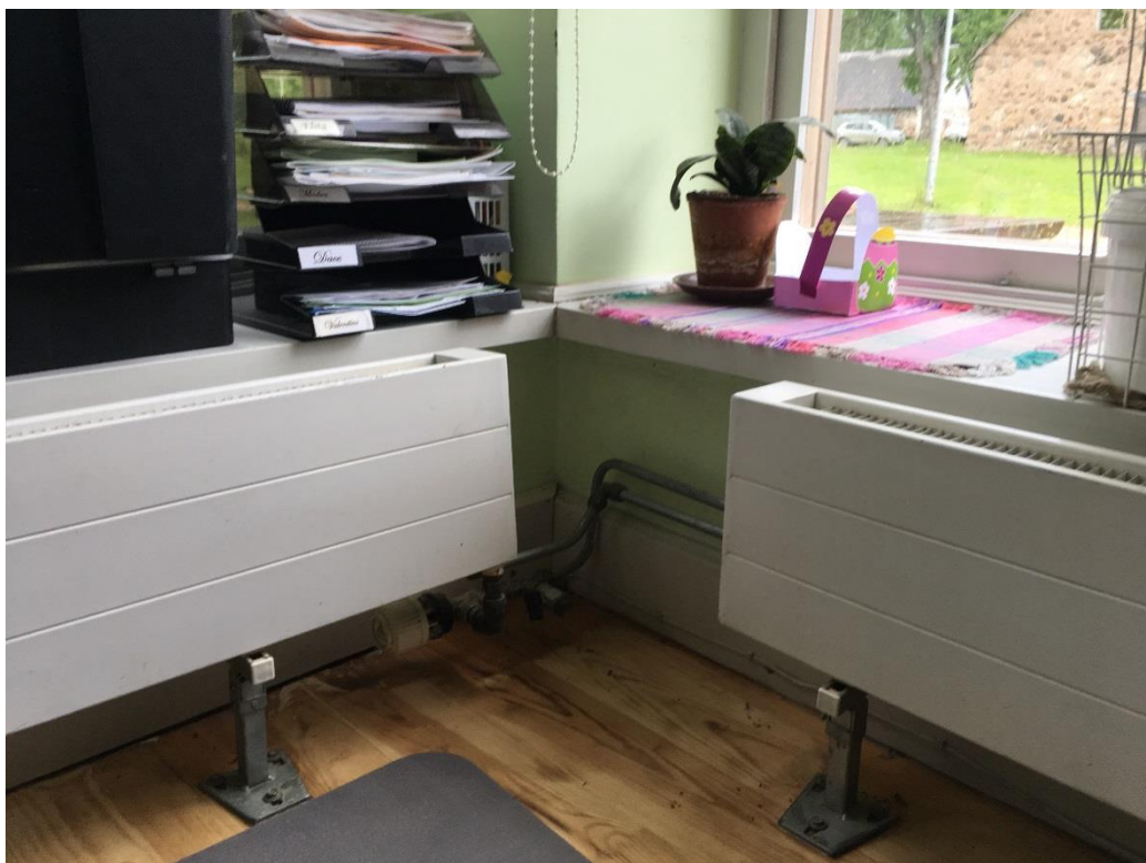
Att. Nr.10 Apkures radiatori ar termoregulatoru
